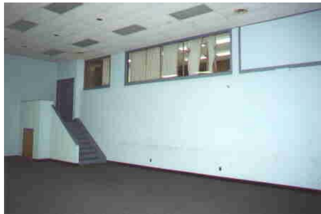
This is a picture of the War Room as it looks today.
