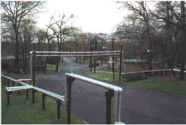
Overhead pipes provided heat and hot water to each building on the base.
